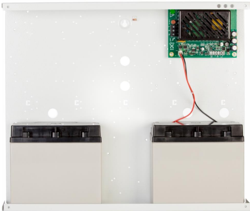
An E-box fitted with a Dycon D1555 5A PSU and 2 x 17Ah VRLA batteries, showing ample space for extra peripherals
